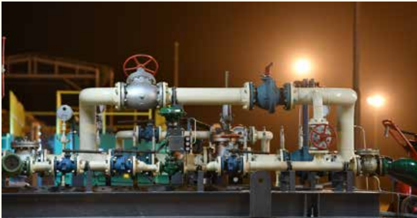
Metering System, Kalabagh Gas & Condensate Field, Punjab
