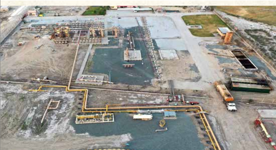
HRL Compression Project, Mari Gas Field, Daharki - Sindh
