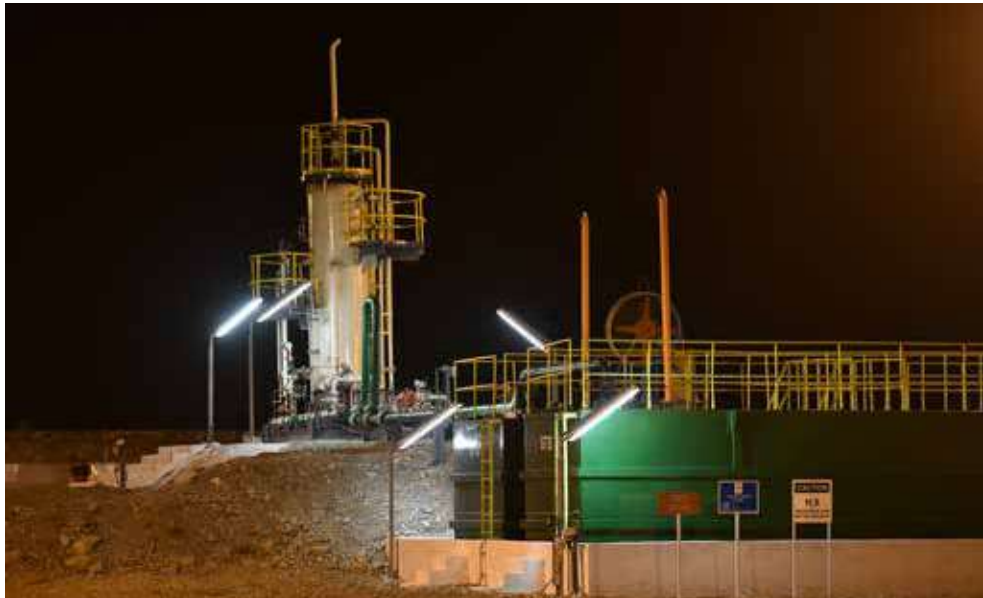
Bolan East Oil Field, Ziarat Block - Balochistan Producing Well 1, MPCL Working Interest 60%, JVP: PPL Europe 40% Production - Oil: 840 BBLs per day
