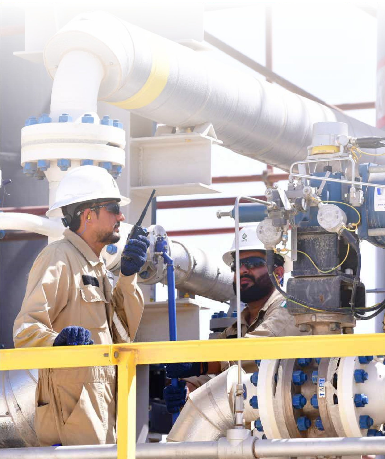
SGPC Plant, Mari Gas Field, Daharki - Sindh
