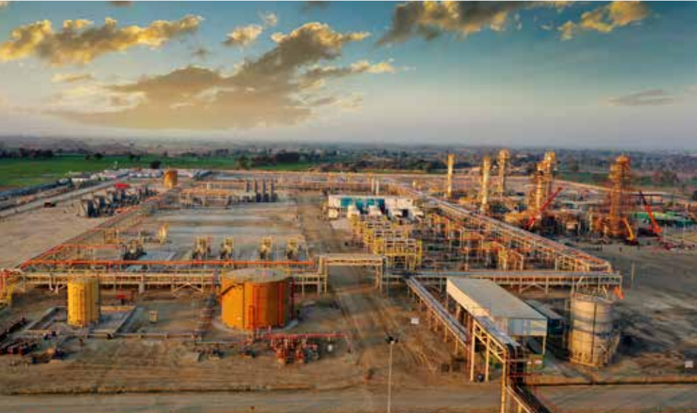
Commissioning of Sachal Gas Processing Complex, Mari Gas Field, Daharki - Sindh
