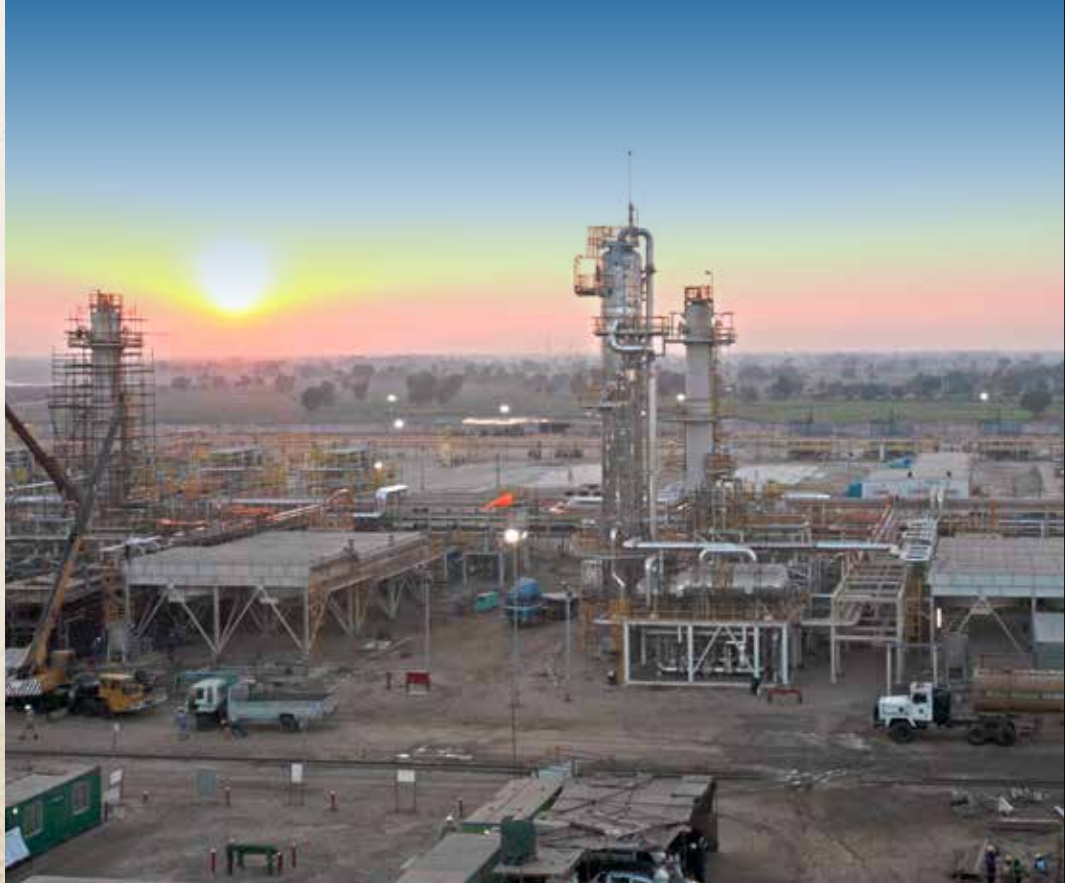
SGPC Plant, Mari Gas Field, Daharki - Sindh
