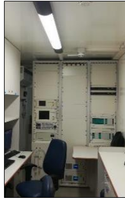
Mud Logging Unit
